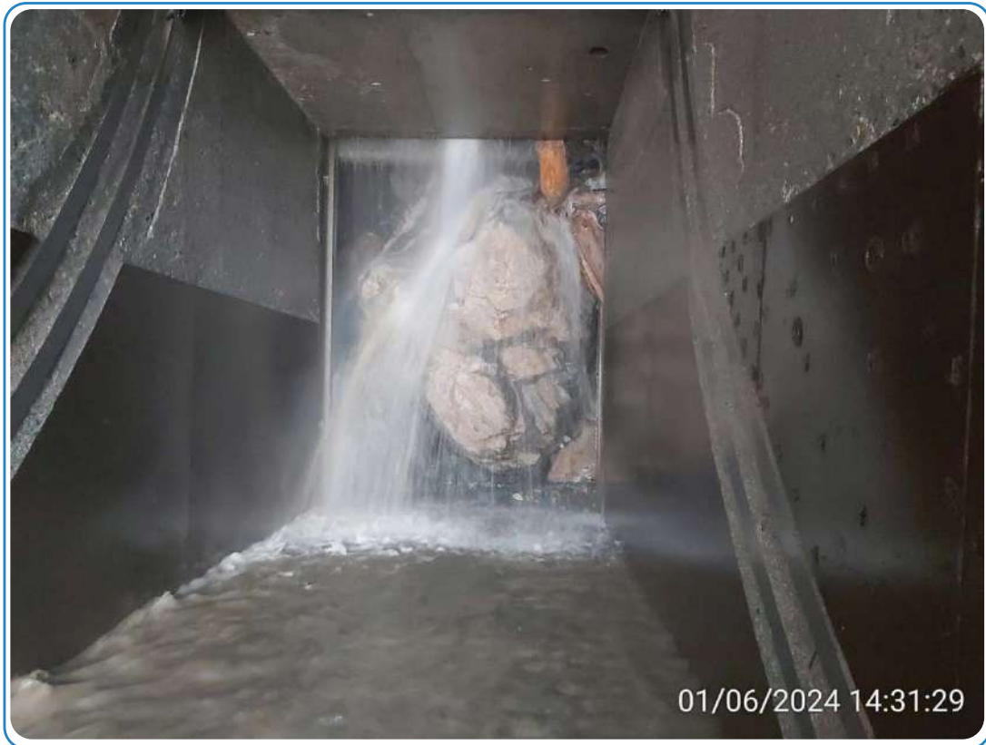
Boulder Blocking Undersluice Way
