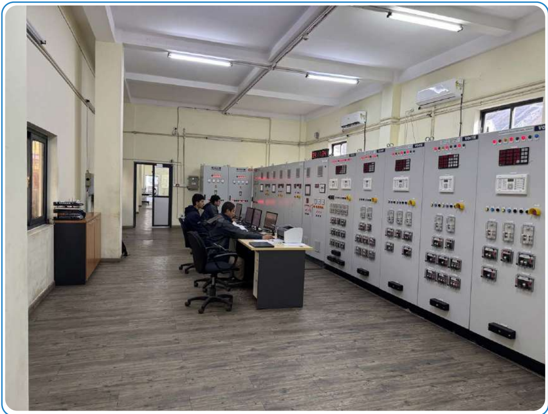
Mistri Control Room
